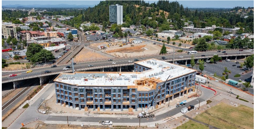
Looking east towards Skinner Butte at construction underway on the first parcel of the Atkins-Dame Downtown Riverfront housing development
