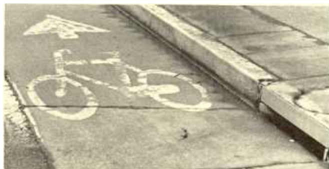
Curb inlets drain away surface water and replace bike-eating metal grates.
