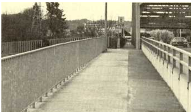
Heavy railing now protects bicycles from cars on City's busiest bridge. Widened sidewalk connects with new ramp.
