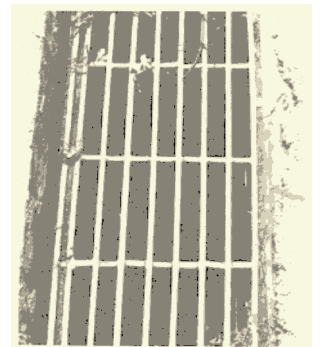
Cross pieces welded to old-style drainage grates prevent bicycle wheels from slipping through.
