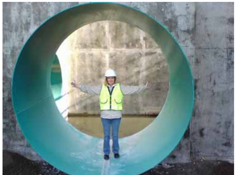
New, large diameter pipe increases peak flow capacity
