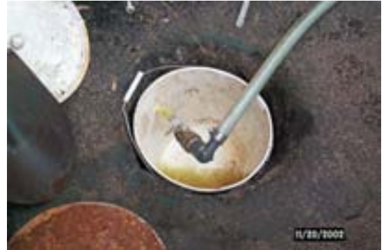
Leachate Bucket with On/Off Valve
